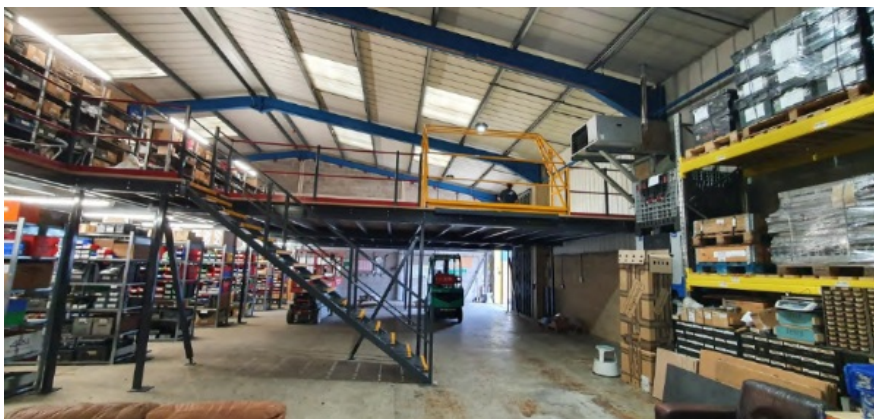
Above: Mezzanine just finished, packing tables beneath and racking above not yet in & on.
